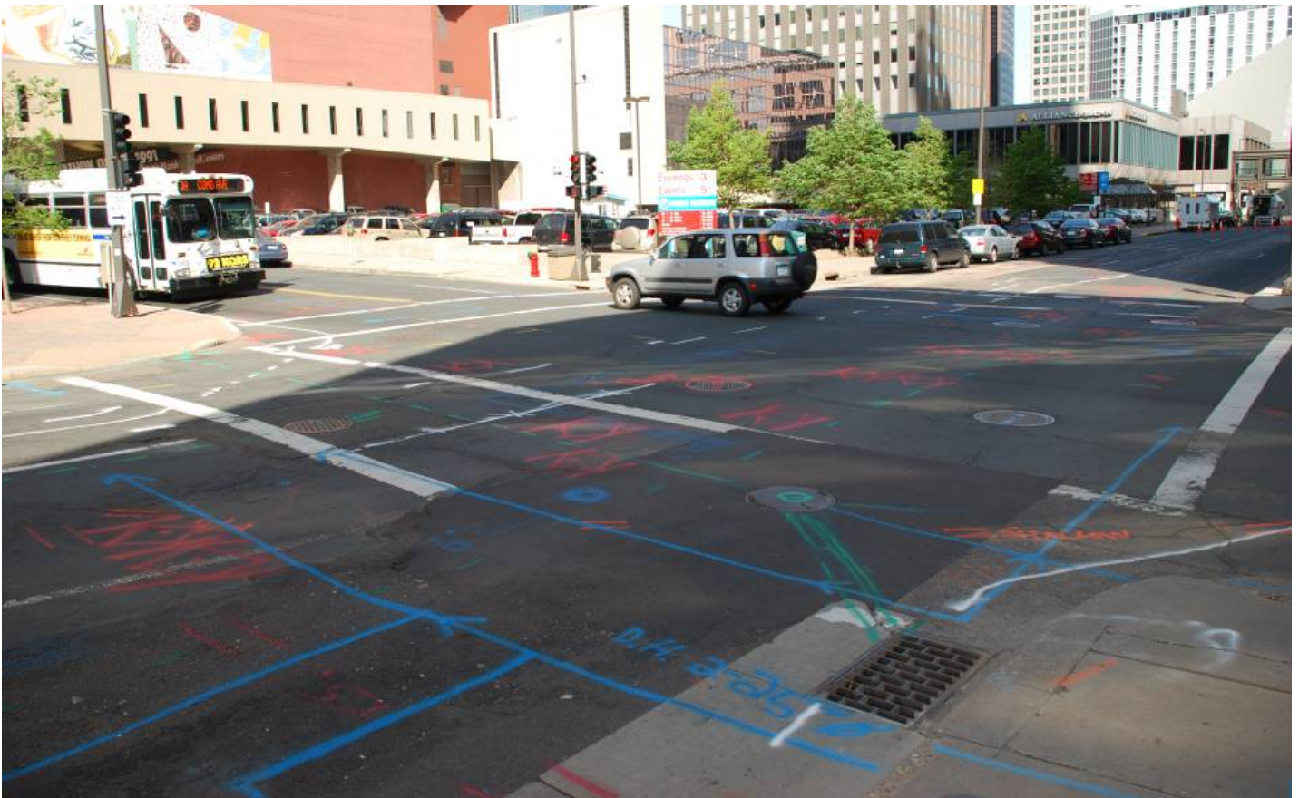
Markings at the intersection of Fourth Street and Minnesota Street identify the location of underground utilities to be relocated in anticipation of Central Corridor LRT.
