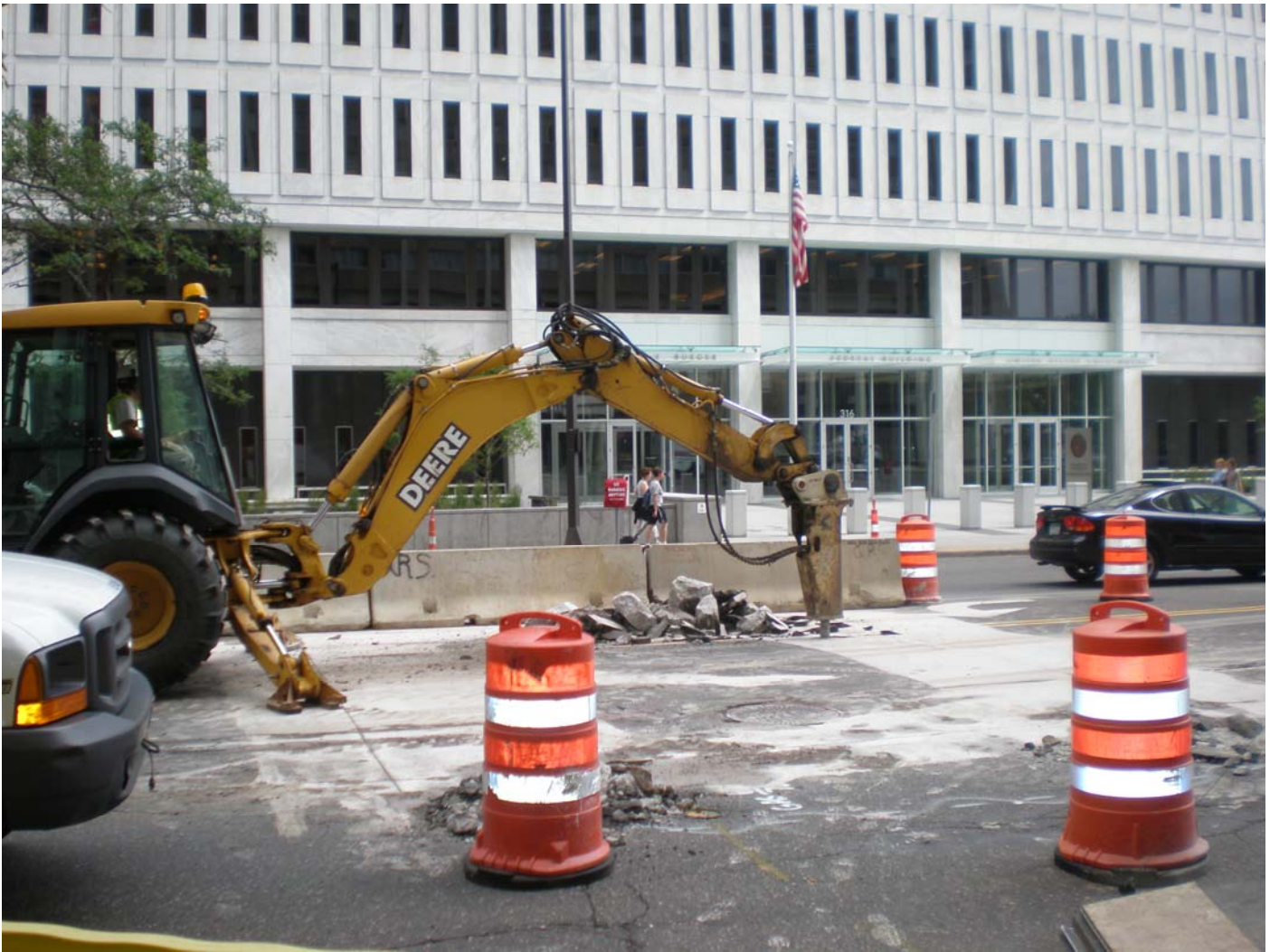
Xcel construction crews use a backhoe with jackhammer attachment to remove portions of the Robert Street road surface to expose existing utilities
