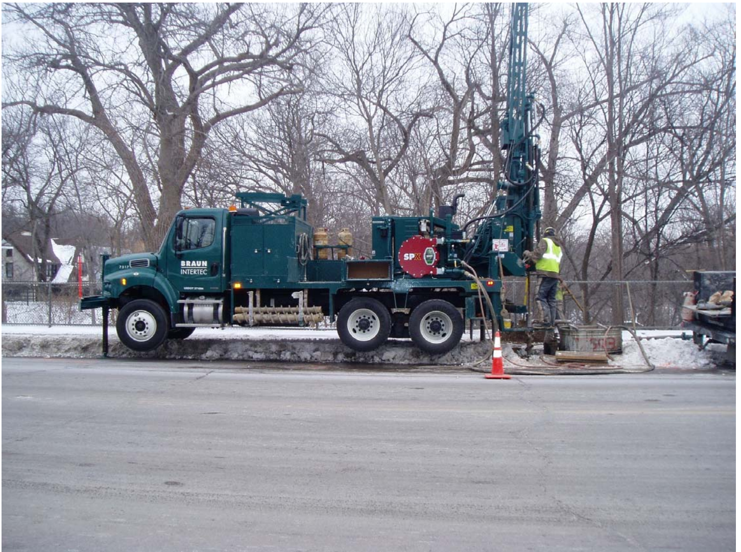
An example of the type of drilling rig that will be used
